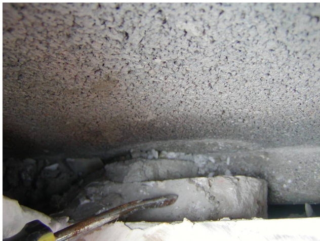
PHOTO 5 - DISINTEGRATION OF GYPSUM (MORTAR) BETWEEN STONE AND BACKUP WALL.
