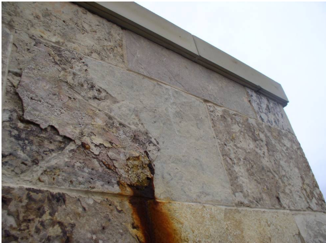
PHOTO 6 - STONE DETERIORATION DUE TO MINERAL DEPOSITS WITHIN THE STONE
