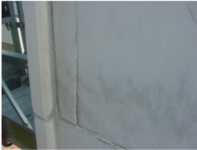
PHOTO 1- FISSURE IN STONE VENEER
