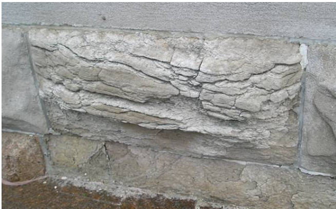
PHOTO 7 - FREEZE-THAW DAMAGE EXACERBATED WITH THE USE OF DE-ICING PRODUCTS
