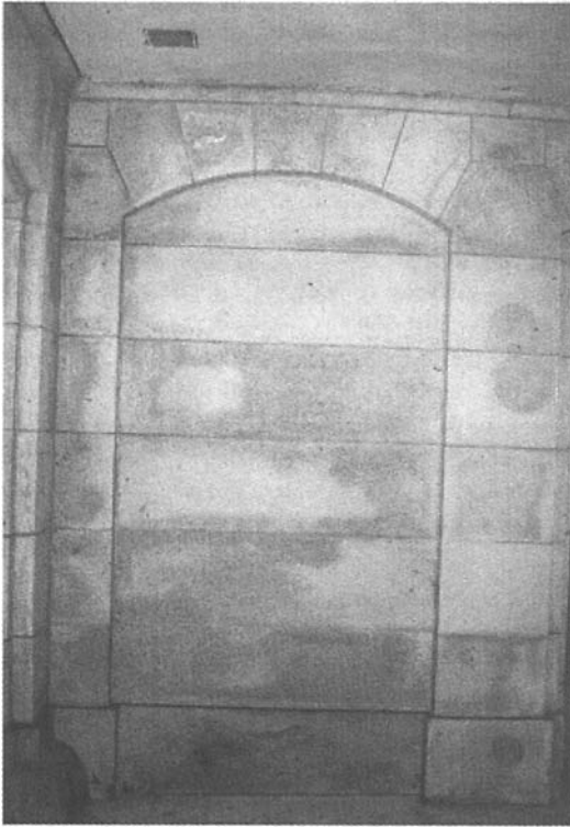
Figure 5 - Heavily mottled granite surfaces below a landing with a history of water leakage problems
