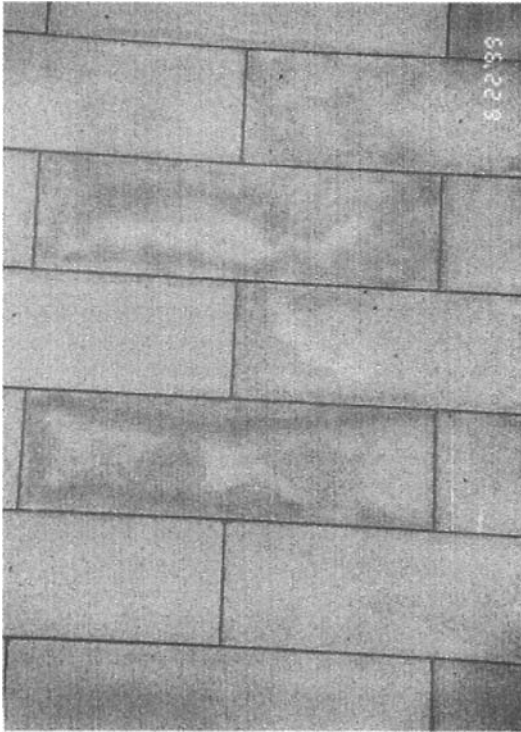
Figure 1 - Typical mottled appearance of the exterior granite surface
