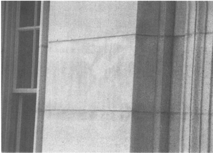
Figure 6 - Pattern of deterioration and dirt accumulation resembles an uneven wash pattern such as would be created by cleaning with an acid soaked rag. Note how the pattern extends from stone to stone
