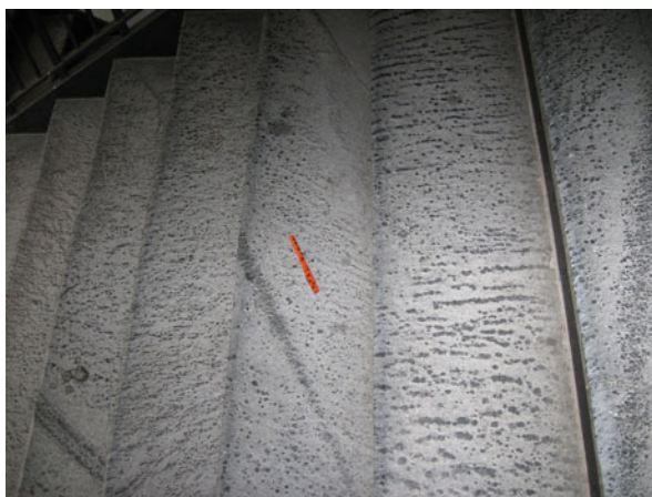
Fig. 3.68 Staircases in the Geology Department at Princeton University (U.S.A.) showing significant abrasion. The staircases are made of an altered and metamorphosed ultramafic rock. The parts that wear down are talc plus magnesite. The more resistant lines and bumps are chlorite and/or pyroxene
